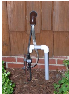
Shack end - Ground Rod and PolyPhaser protection
